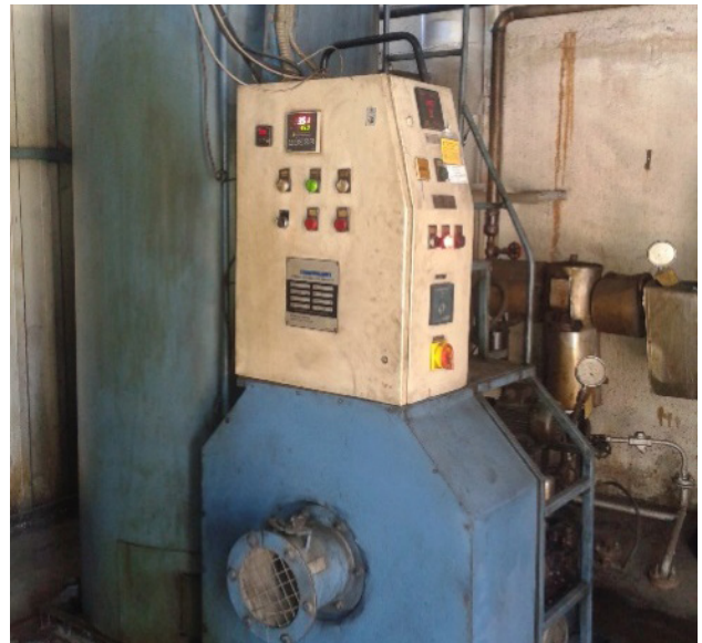
Biodiesel based boiler at Nashik
