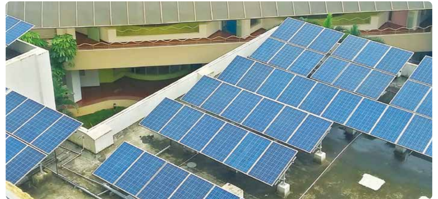
Rooftop solar plant at our Mahape R&D Center
